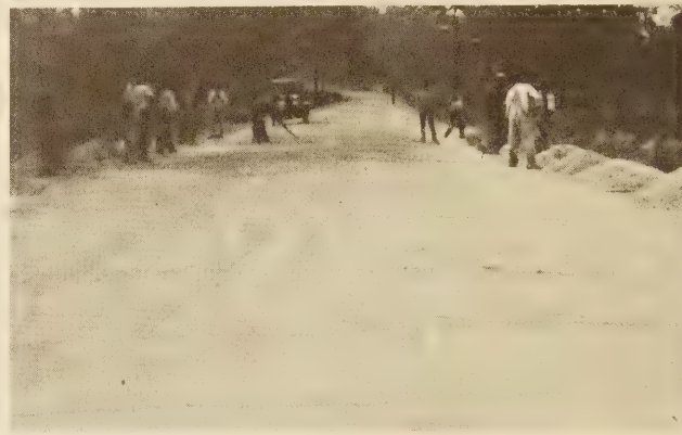
FIGURE 4.—SPREADING THE COARSE STONE ON THE FINE STONE CUSHION. THIS SECTION, EXPERIMENT 2-C, WAS CONSTRUCTED WITH ASPHALT EMULSION BY A MODIFIED PENETRATION METHOD
